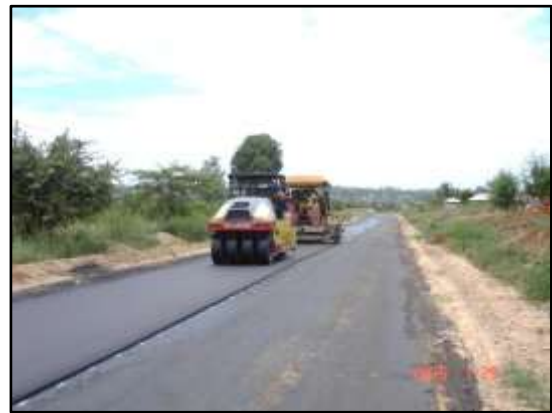
Photograph 6 Surfacing of the recycled base after being opened to traffic for two months
