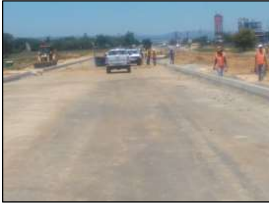
Photograph 3 Condition of the exposed sub-base after 3 months of heavy rains
